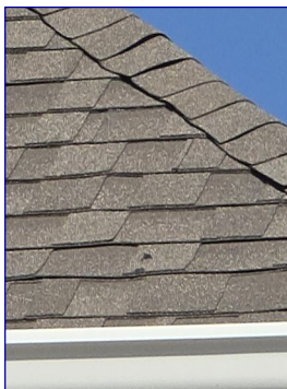
Damaged asphalt shingle on southeast corner of roof
