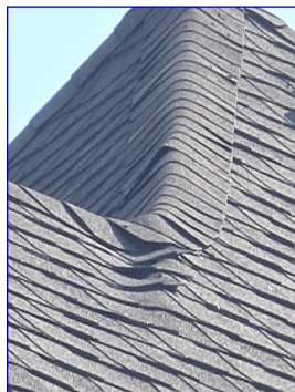
Possible raised shingles
