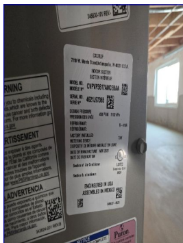
Furnace data tag
