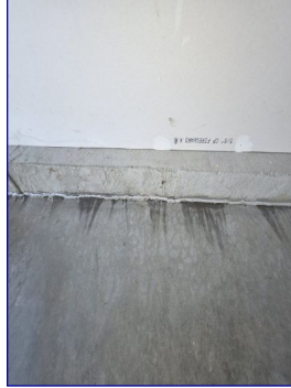
Signs of water intrusion on garage floor
