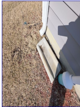
Southwest gutter downspout splash guard not in place
