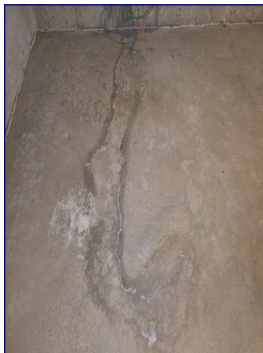
Efflorescence on concrete basement floor
