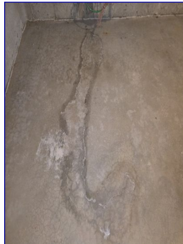
Efflorescence on concrete basement floor
