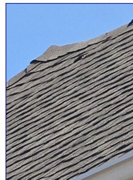
Possible raised shingles
