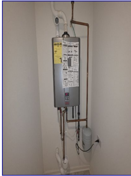
On demand water heater
