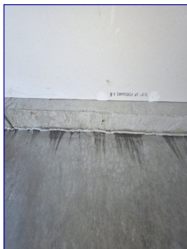
Signs of water intrusion on garage floor
