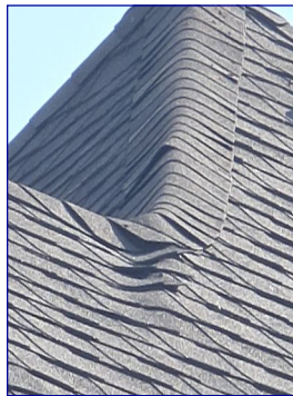
Possible raised shingles
